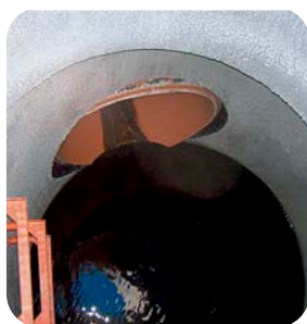
Lack of watertightness in concrete manholes
