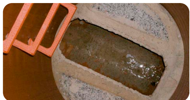
Inside manhole with watertight base
