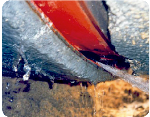
Joint leakage in concrete pipe
