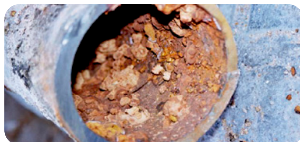
Sewage pipe with material deposits
