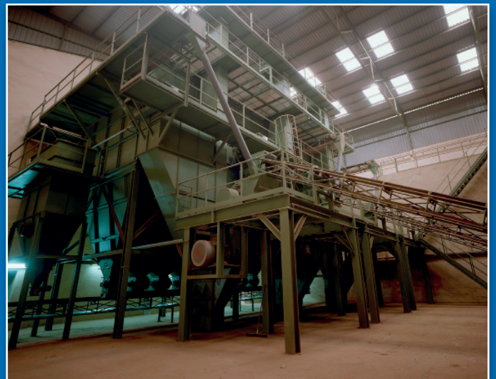
Cintas, molinos trituradores / Conveyor belts, shredders
