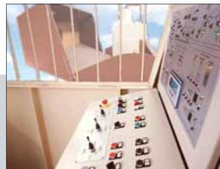
quadro comandi | control panel
