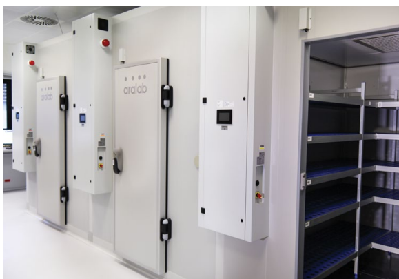
STABILITY ROOMS TURNKEY PROJECT BY ARALAB
