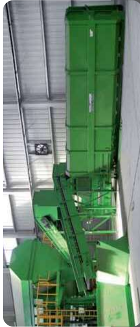
STP-CK with conveyor system
