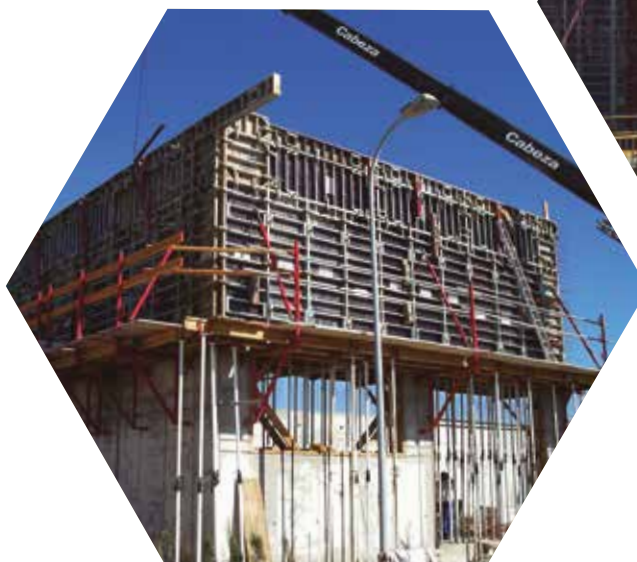
Alicante Desalination Plant, Spain
