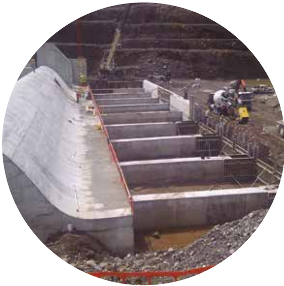
Bocalatun Hydroelectric Power Plant, Panama
