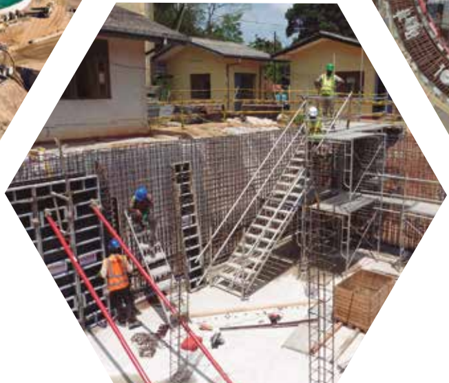
Manila WWTP, Philippines
