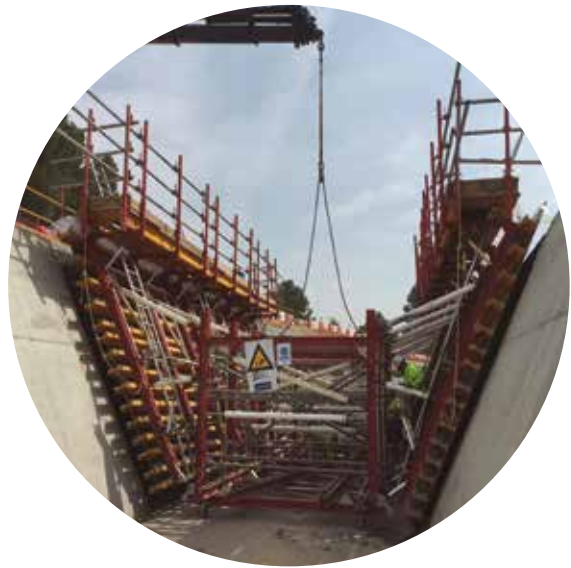
Asco Hydroelectric Power Plant, Spain
