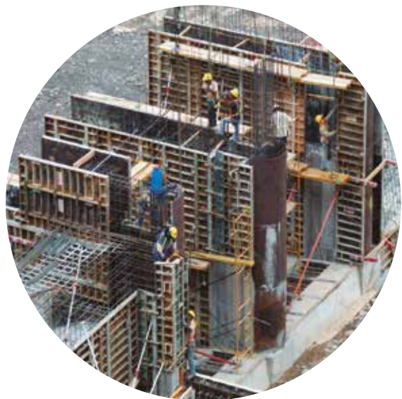
Macho River Hydroelectric Power Plant, Panama
