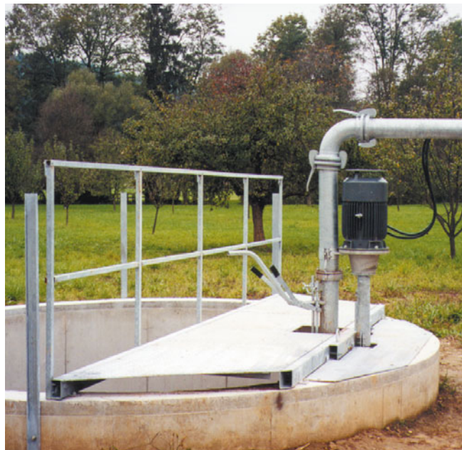
Permanently installed LE model used for transfer
