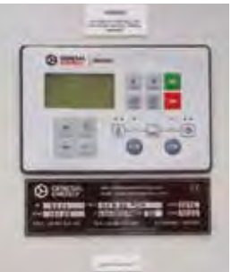
Panel de control
