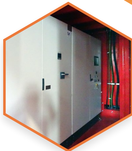
Electrical Room with Control Panel
