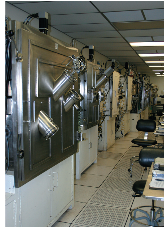
Coating chambers at our Saxonburg facility.
